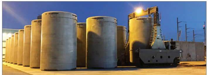
Top photo: Transport of 24th MAGNASTOR system to Kewaunee ISF-SI pad. Bottom Photo: NAC MAGNASTOR spent fuel casks in storage at the Kewaunee ISFSI.
