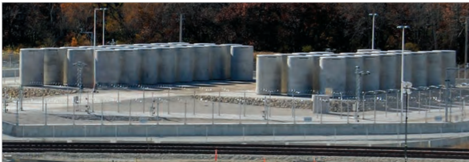
Top right photo: Cask temperatures are continuously monitored at the ISFSI. Bottom photo: NAC MAGNASTOR spent fuel casks on the Zion ISFSI pad.
